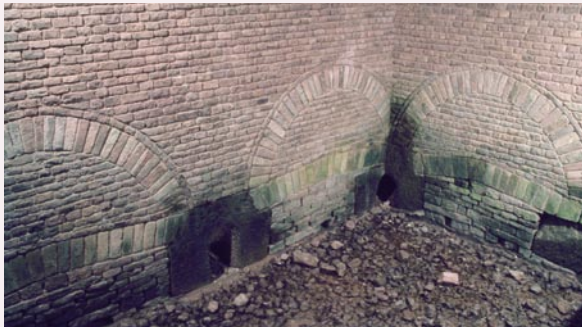
Brunnenstube in Mechernich-Kallmuth
